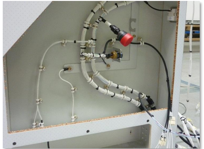
Wiring detail rear side
